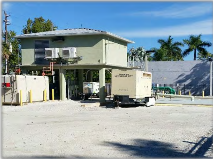
Master Lift Station D – Gulf Bay Road
