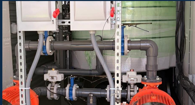
Membrane / polishing skid
