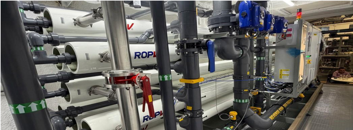
The Valhalla system uses controlled hydrodynamic cavitation (CHC) within a modular treatment train.
