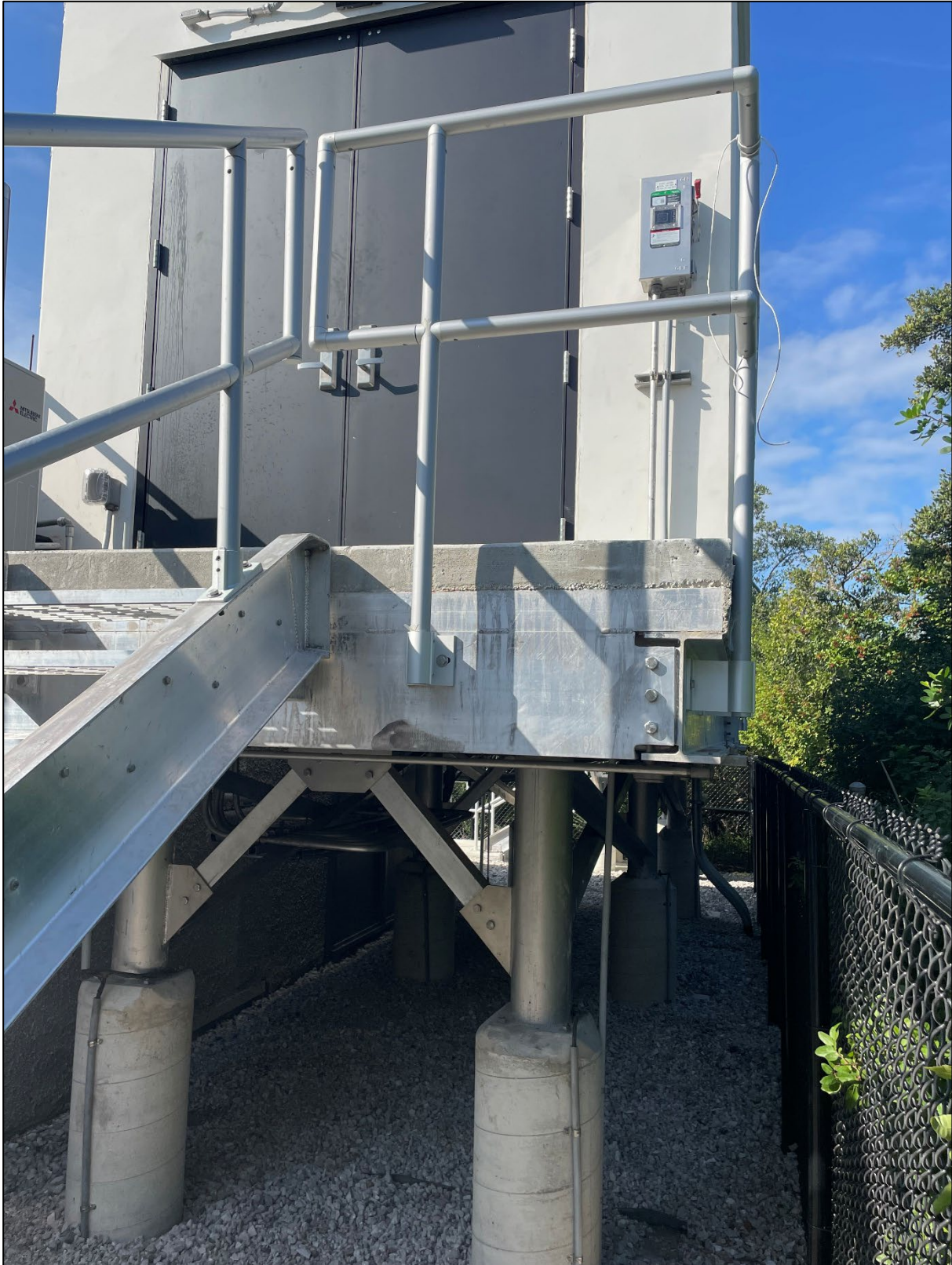
Figure 2: Rear Setback Encroachment
