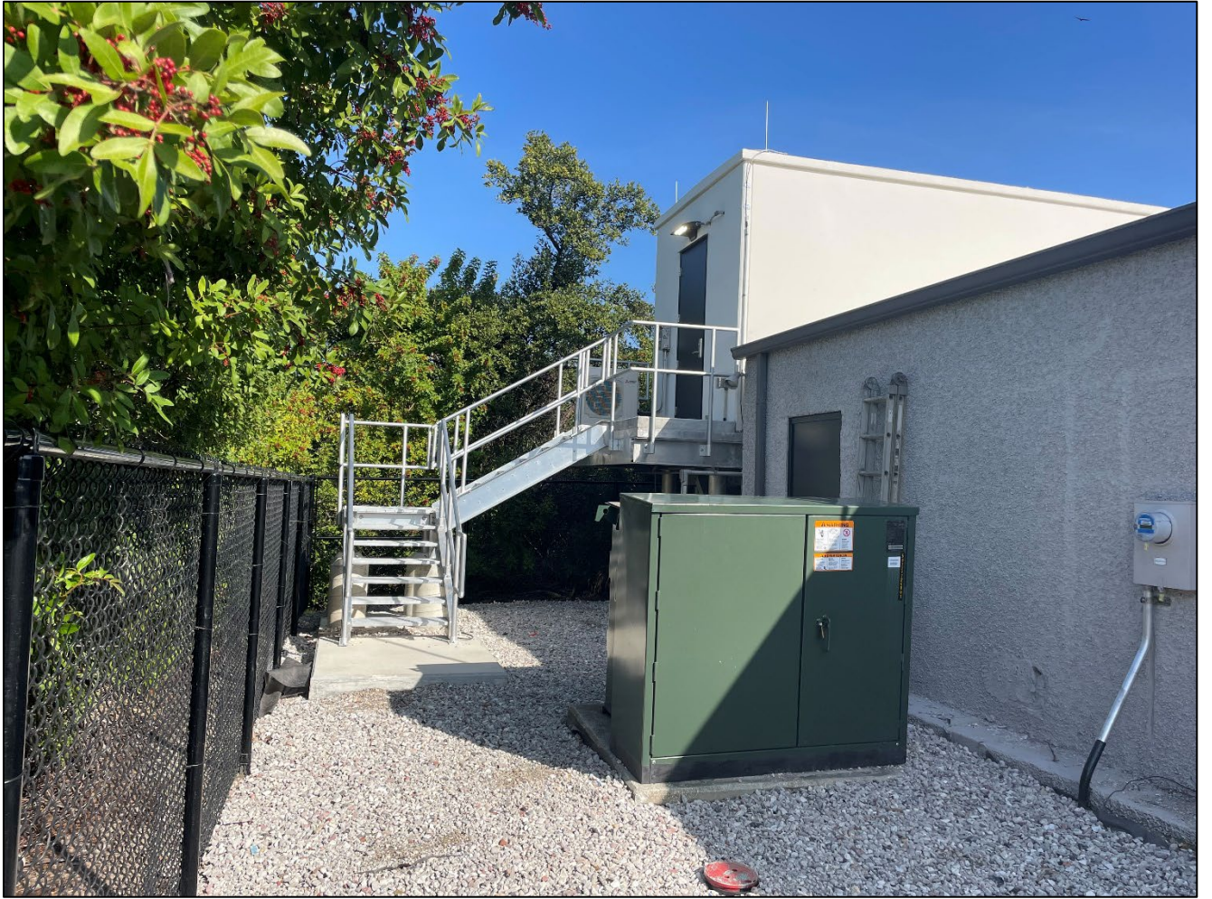
Figure 3: Side Setback Encroachment
