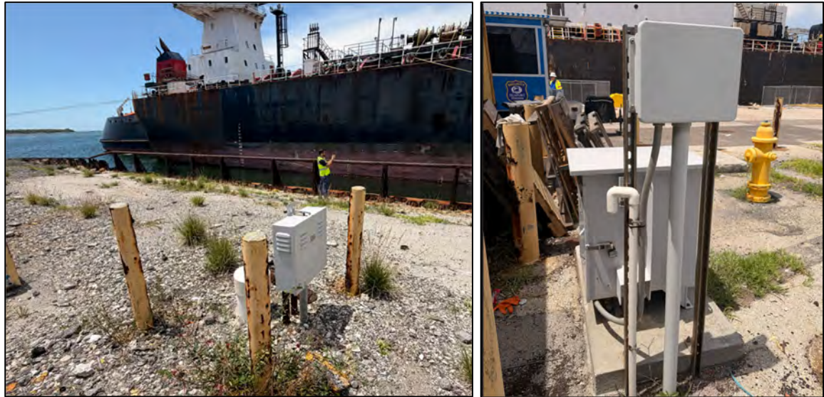
Figure 1: Impressed Cathodic Protection System Components on Berth 10
