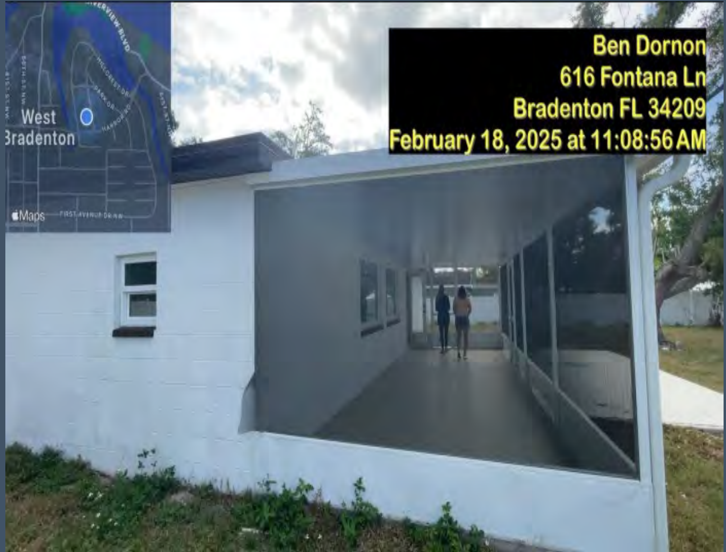
Unpermitted screen porch – looking South
