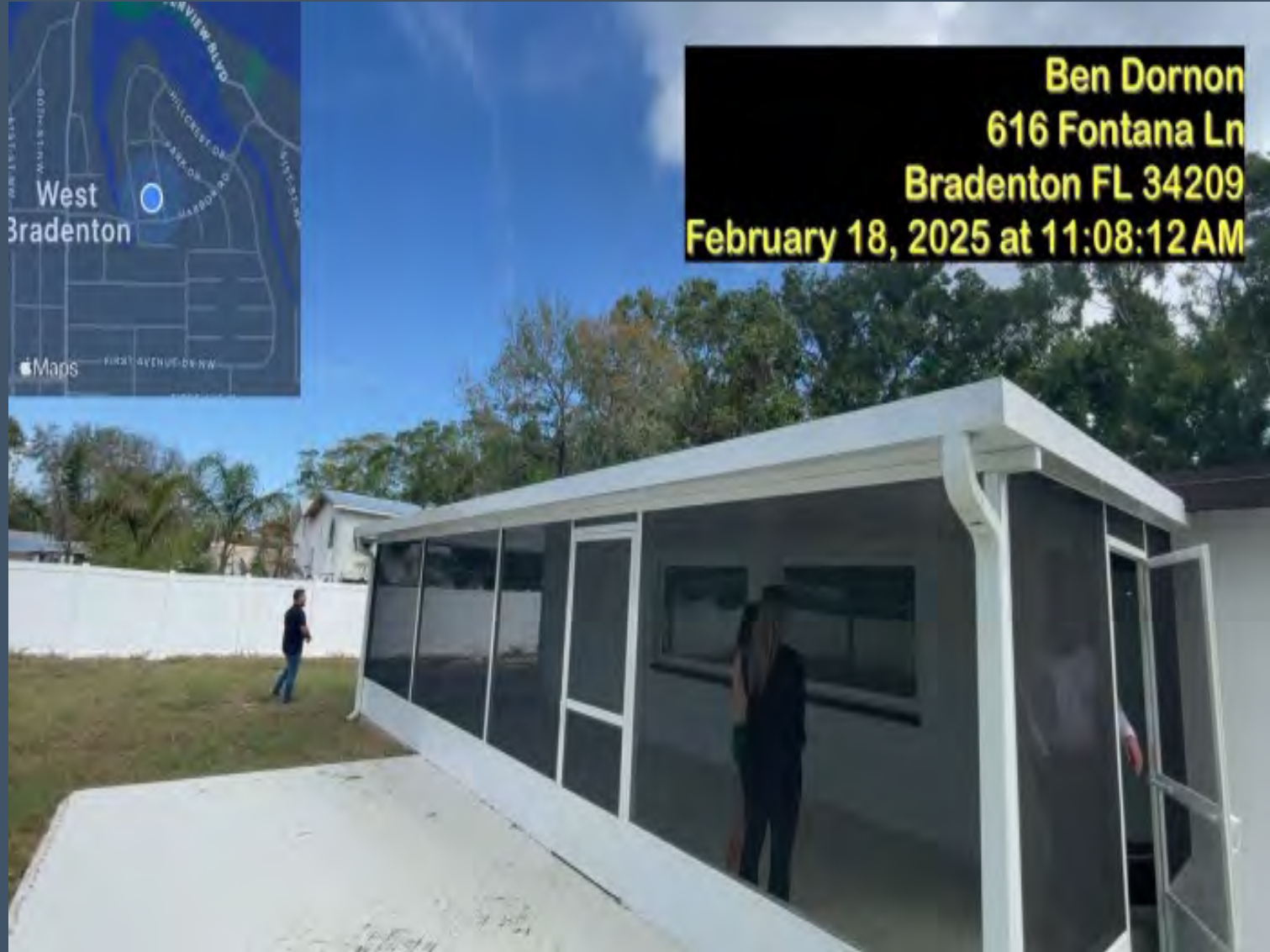
Unpermitted screen porch – looking Northeast
