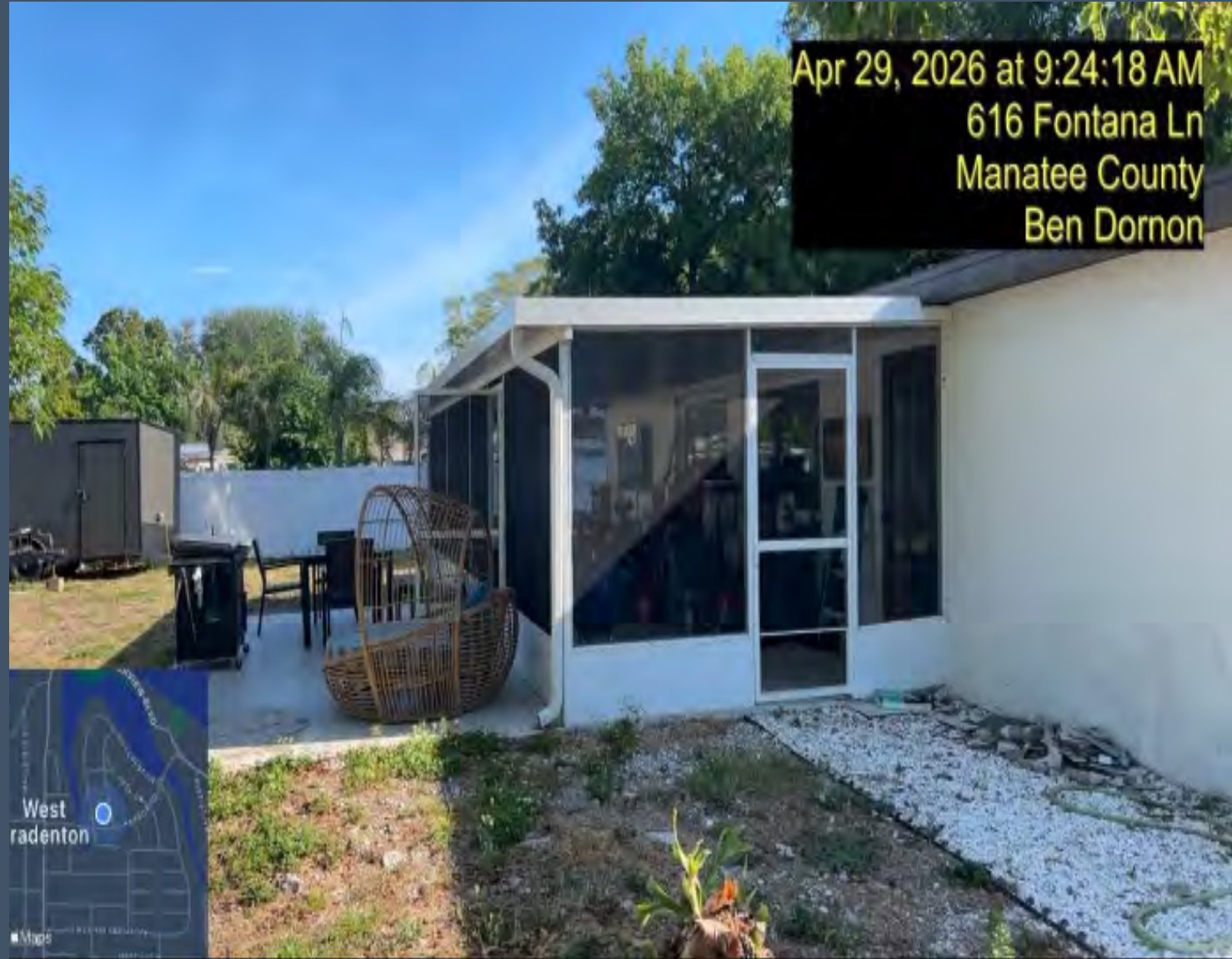
Unpermitted screen porch – looking North
