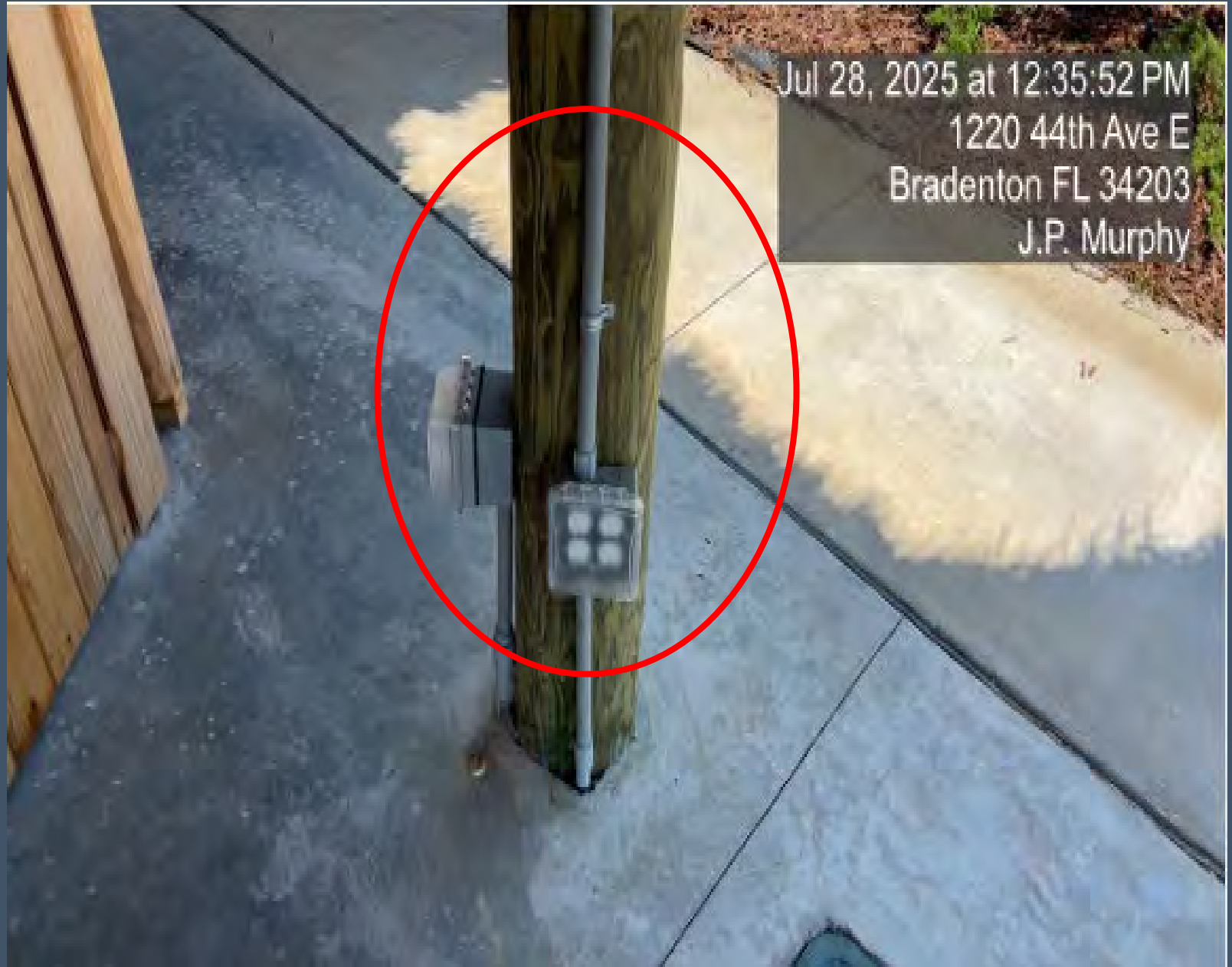
View of the electrical from the property.
