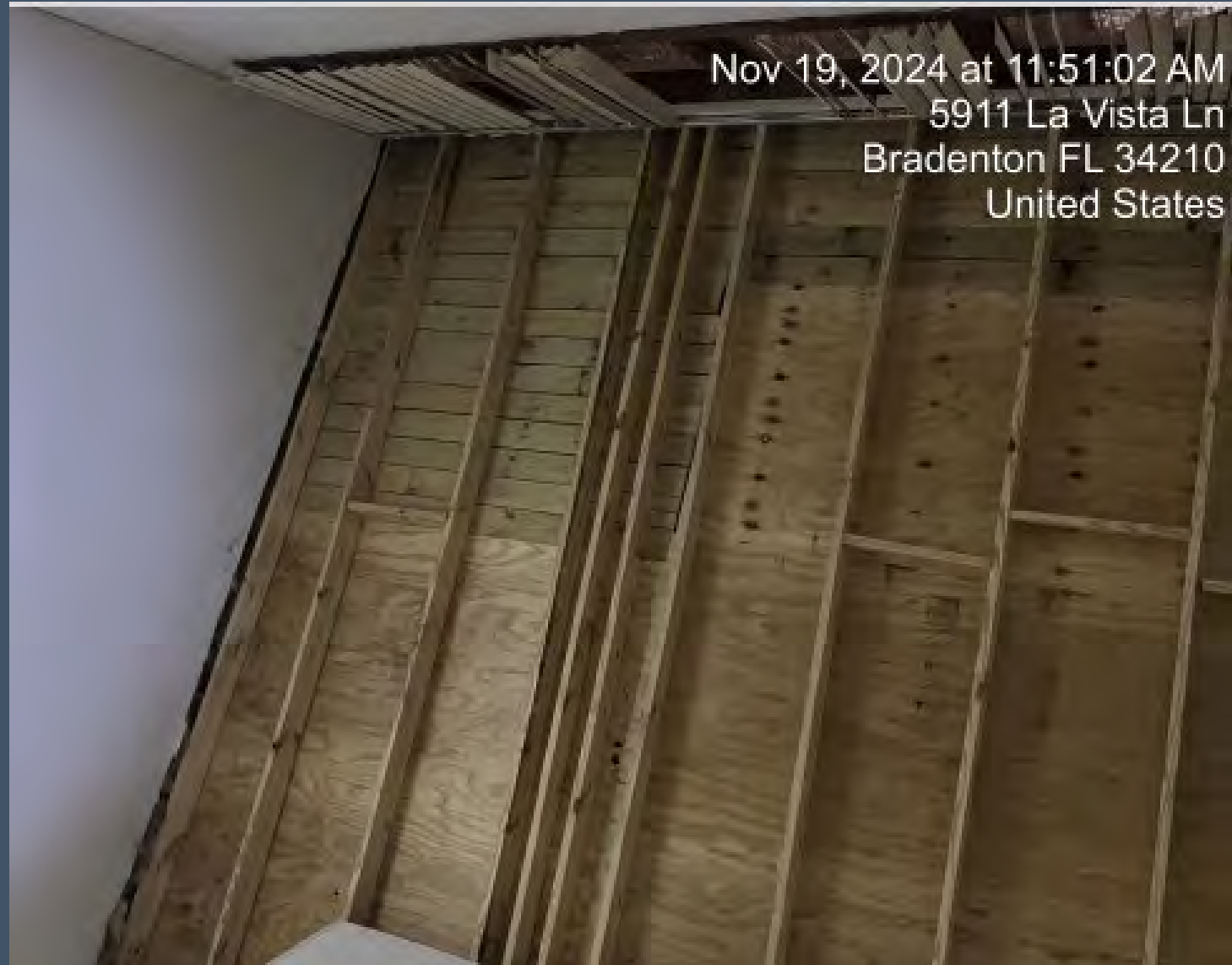
Inside view of unpermitted roof repairs
