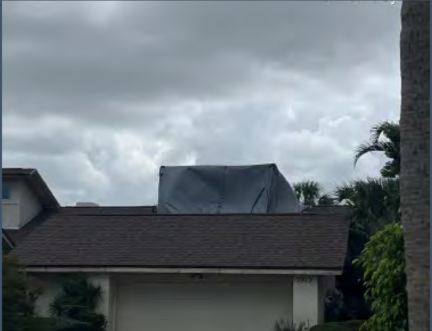
View from street of unpermitted roof repairs
