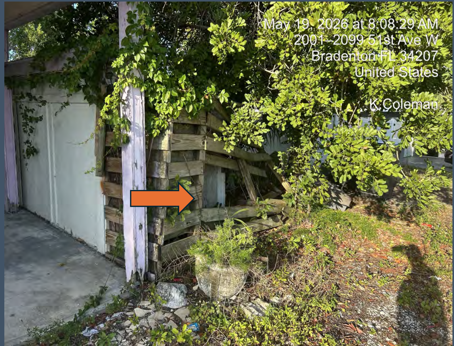
Update view of fence damaged
