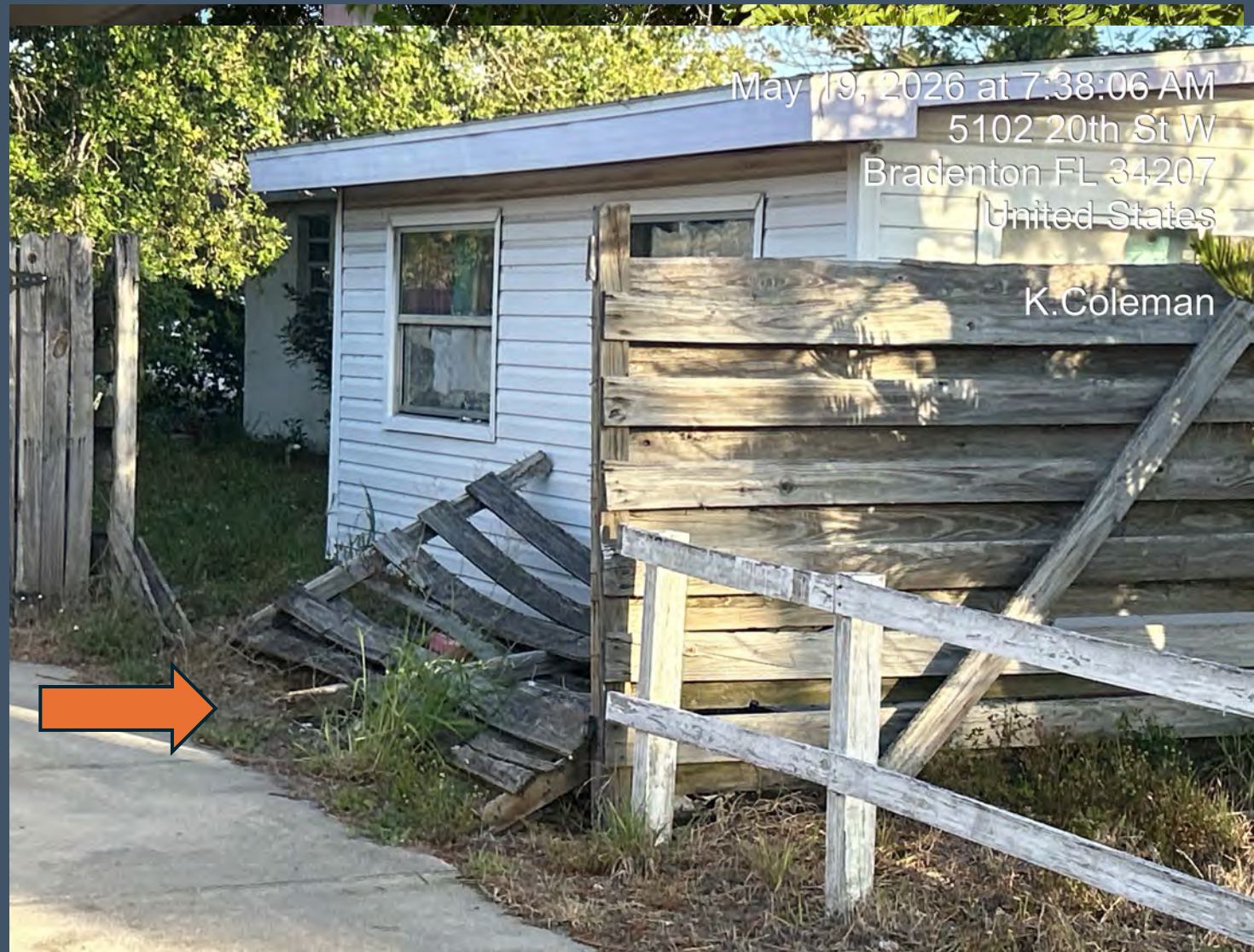
Update view of fence damaged
