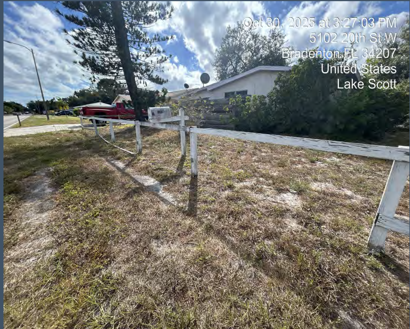
View of fence damaged
