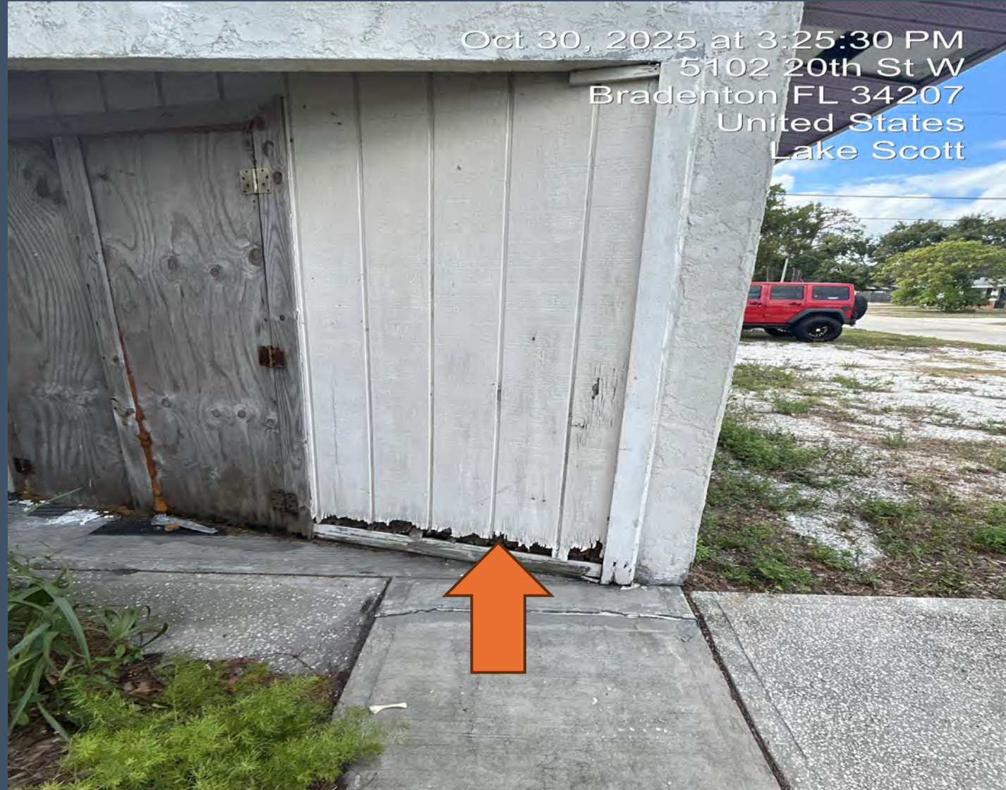
View of siding damaged
