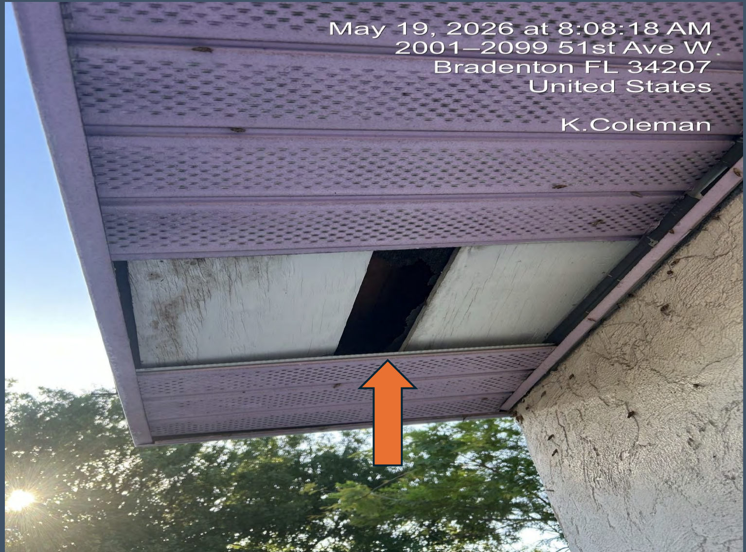
Updated view of soffit in disrepair
