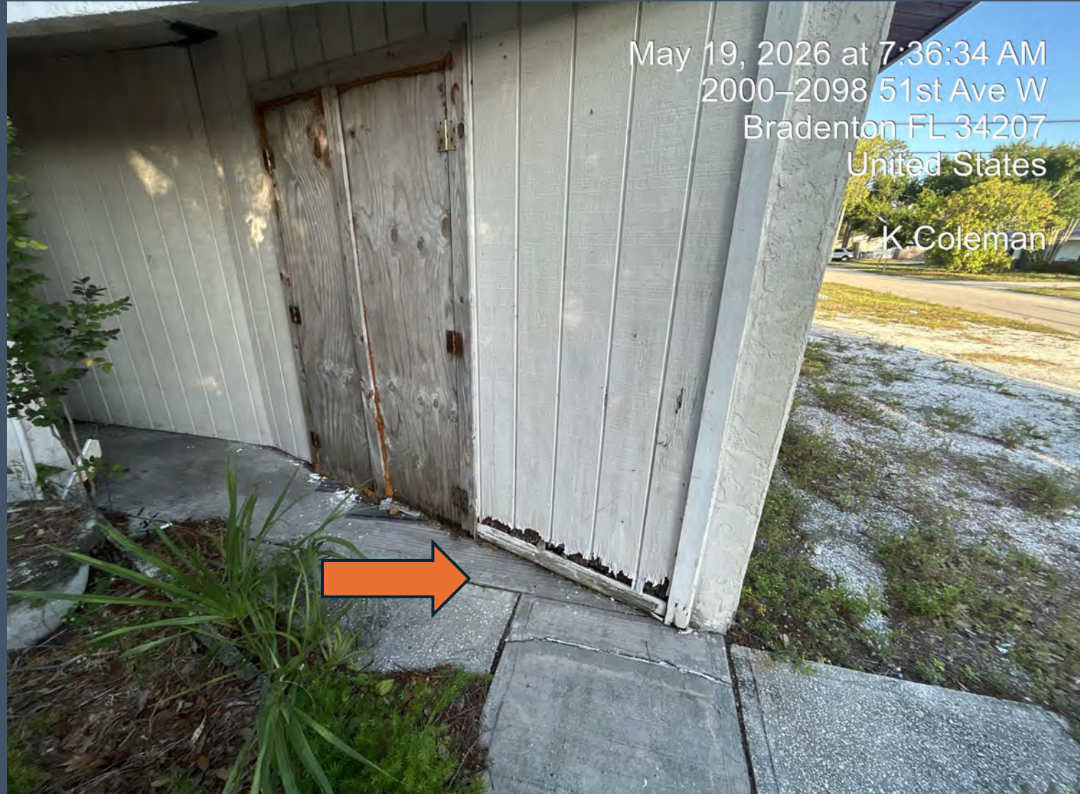
Update view of rotten wood on garage
