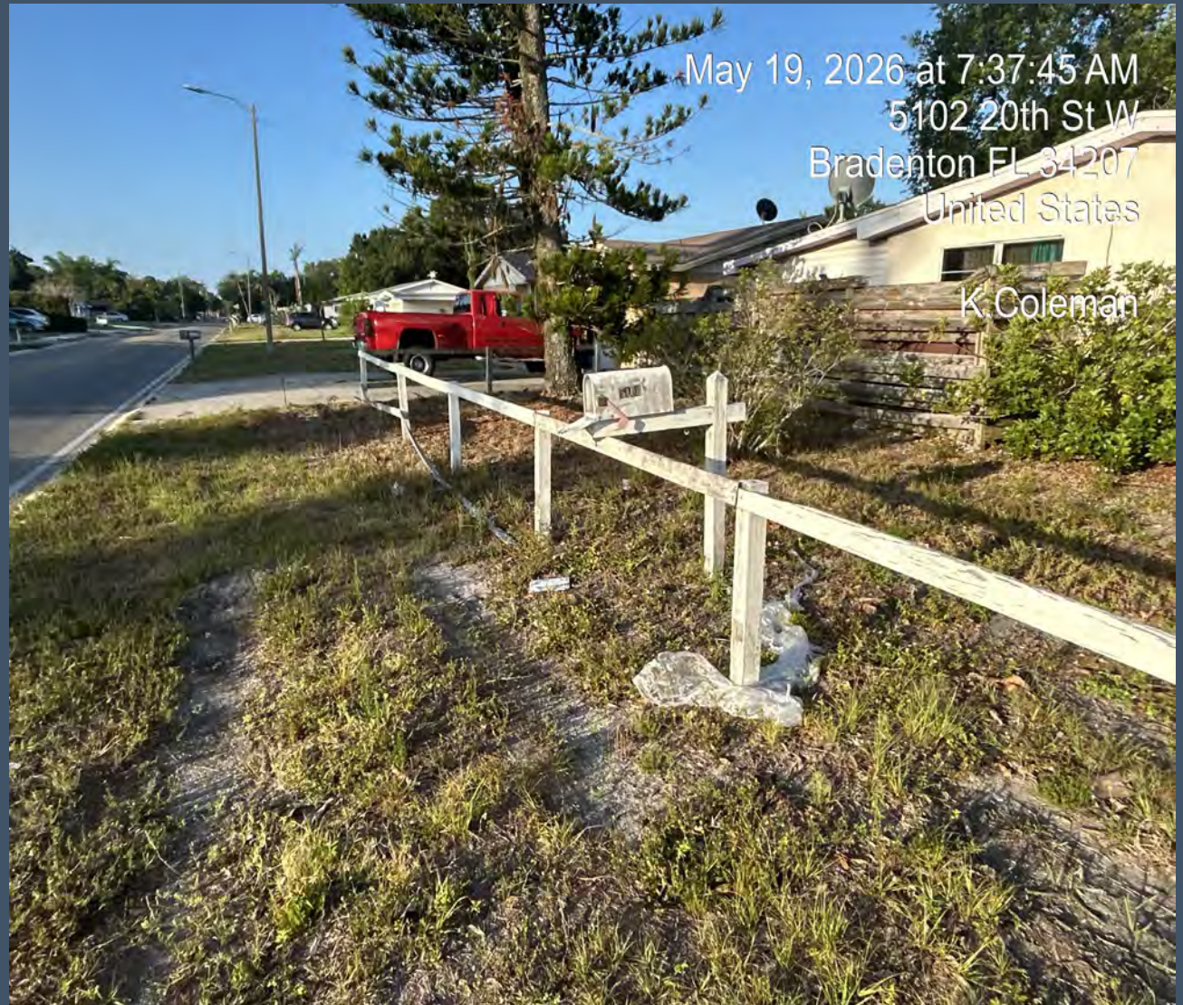
Updated view of damaged fence
