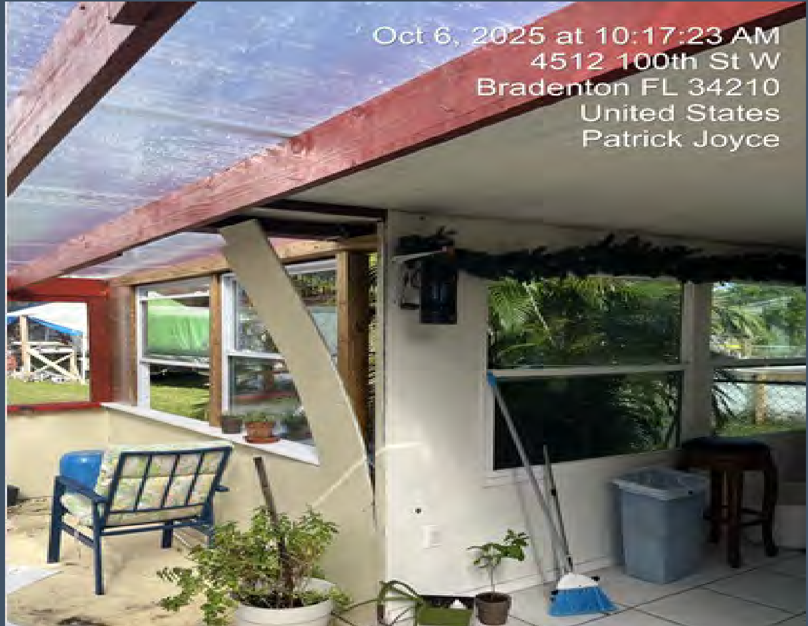
Windows that were added to the unpermitted pool cage
