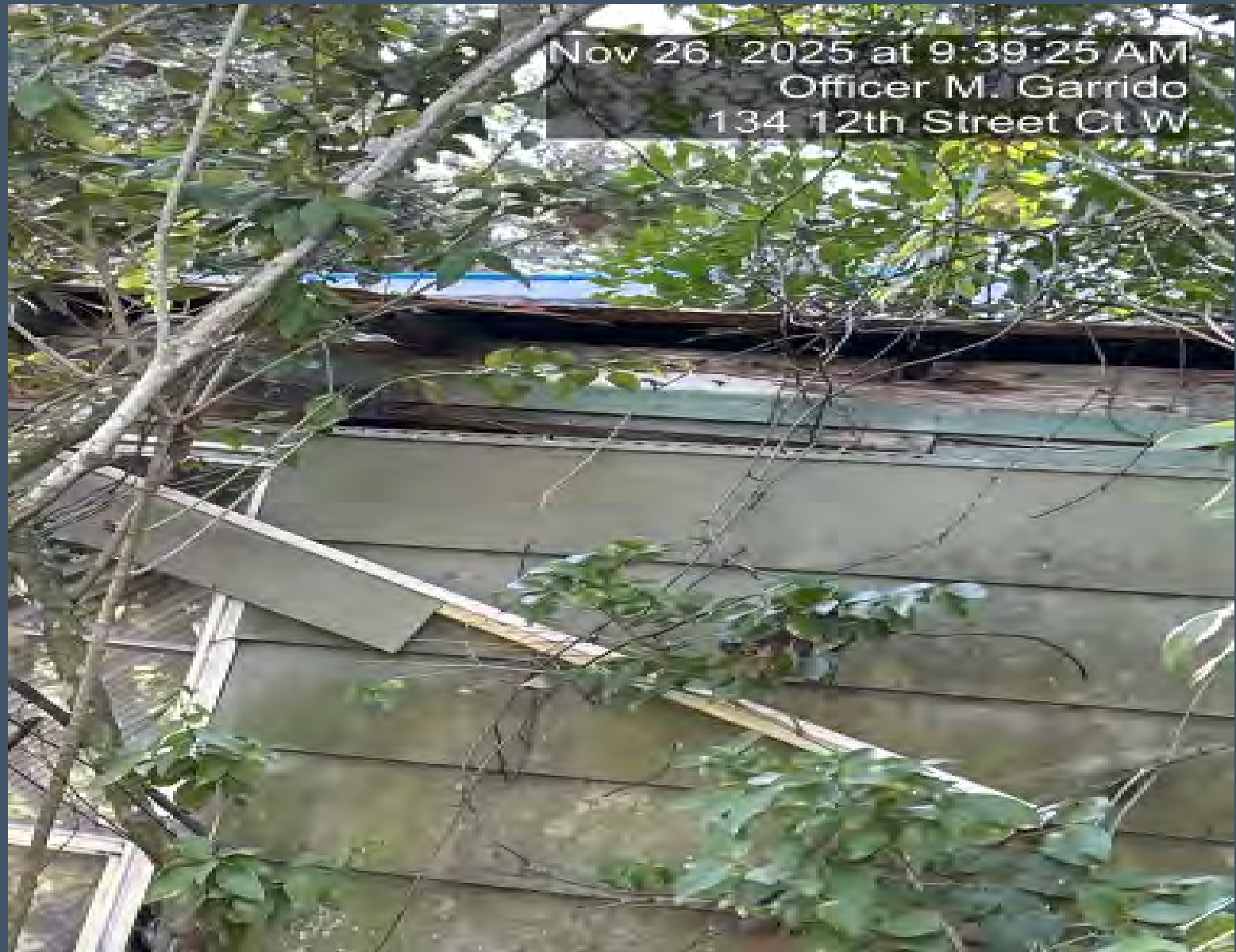
View of the roof from the north (rear) side of the property.
