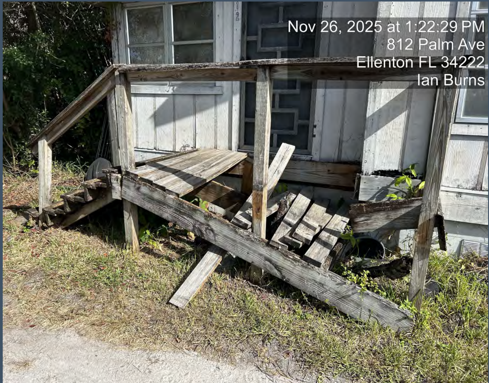
Photo depicts the stairs in disrepair
