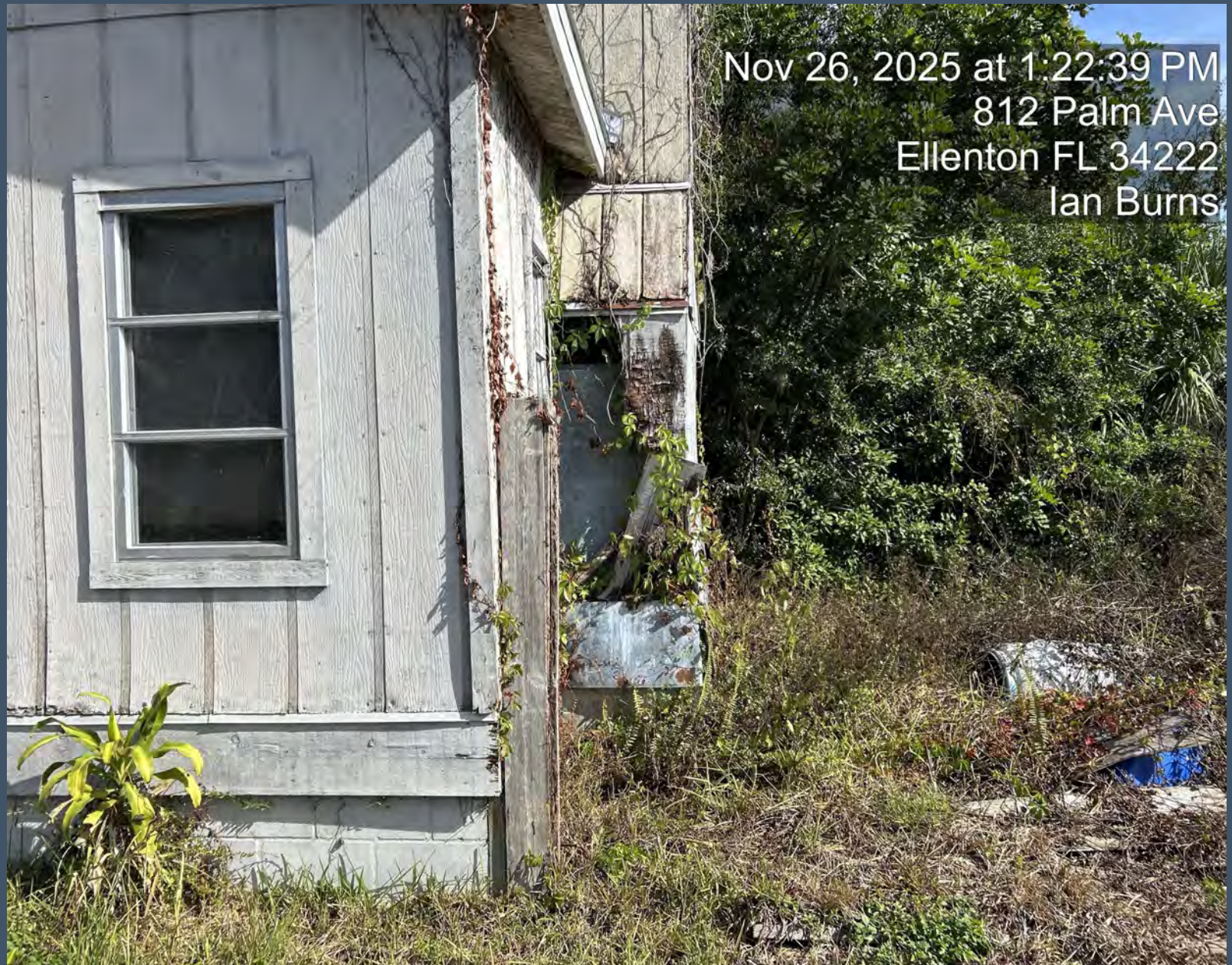
Photo depicts another angle of the side that is in disrepair
