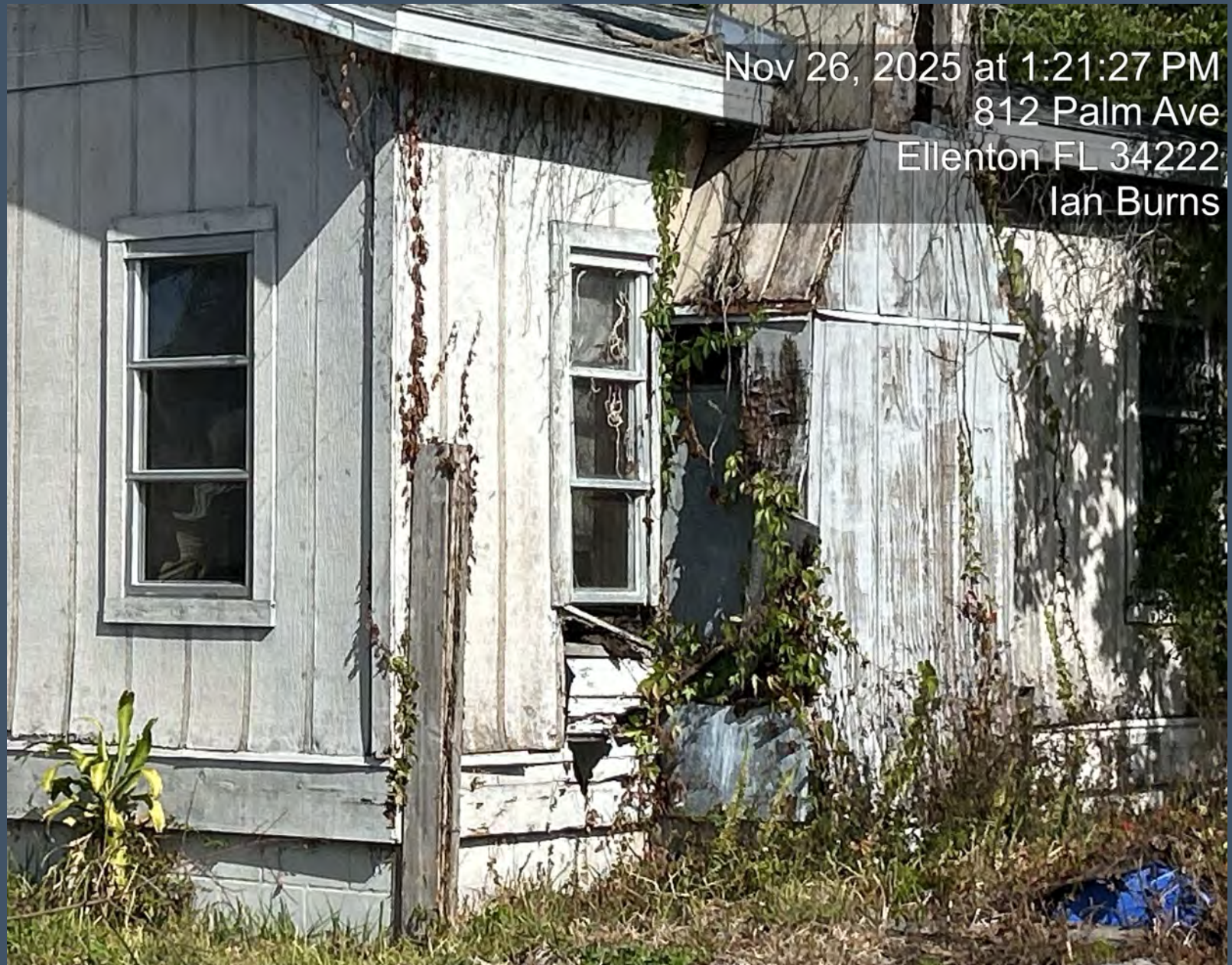
Photo depicts the side of the home in disrepair
