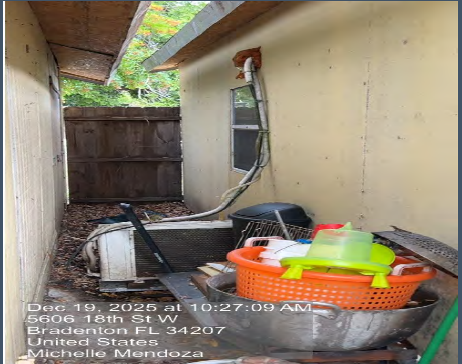
Photo of the AC unit connected to the structure.
