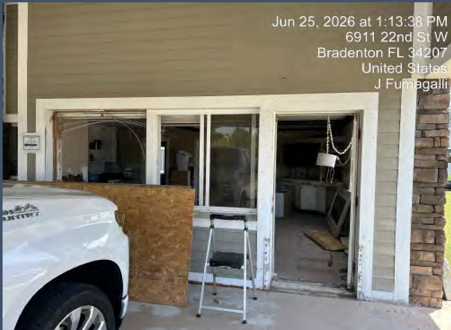
Broken windows in the front of the home
