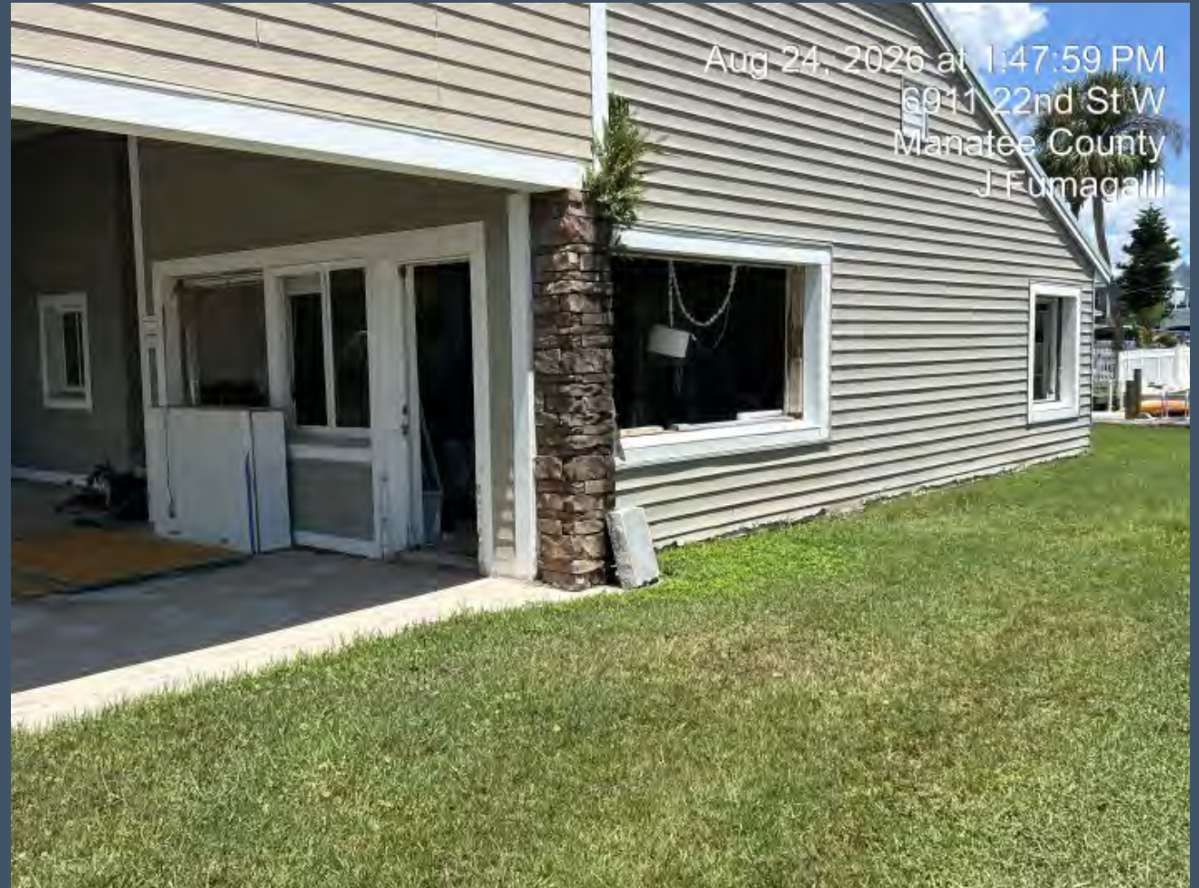
Broken windows on the side and front of the home.
