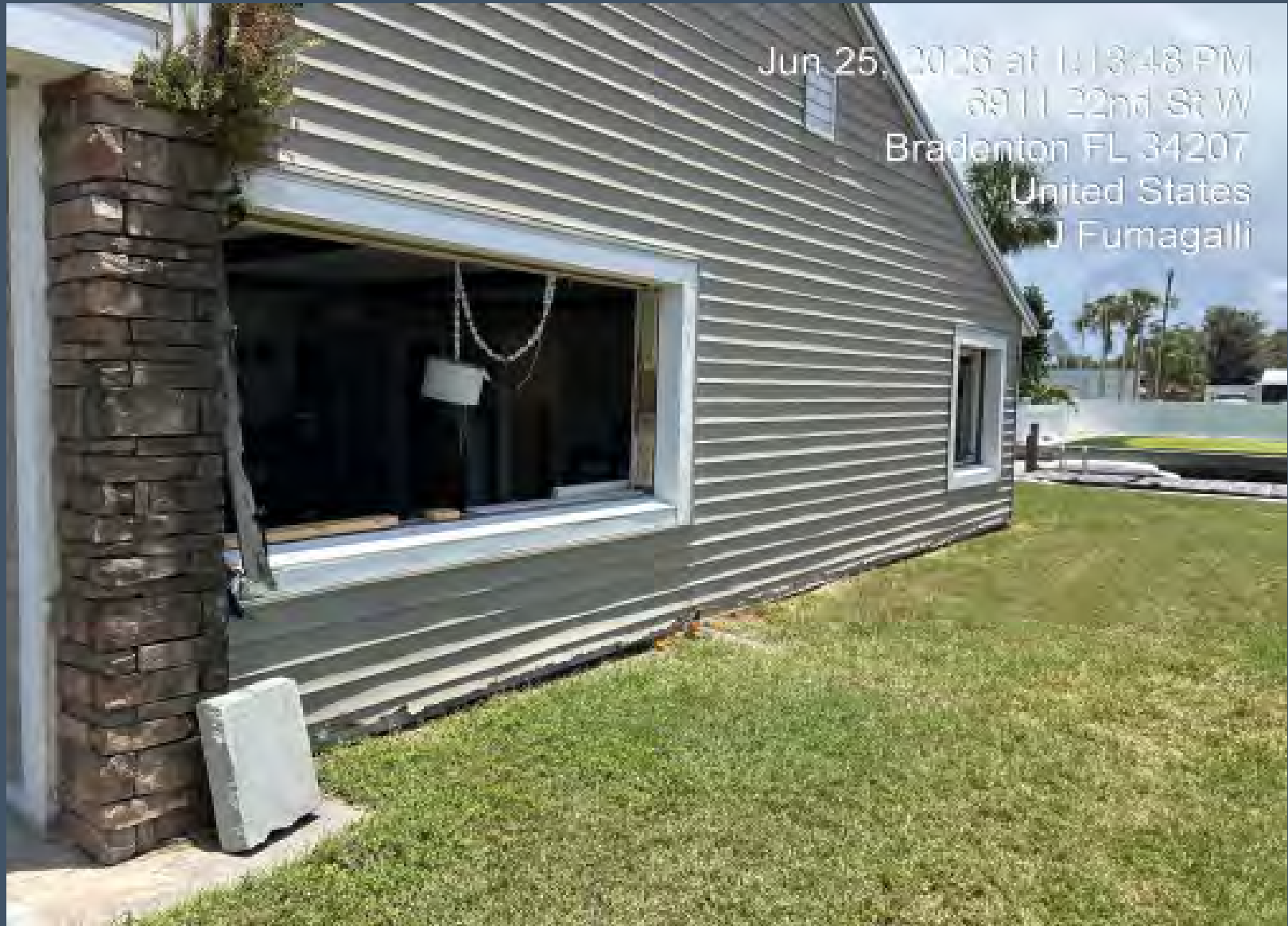
Broken windows on the side of the home
