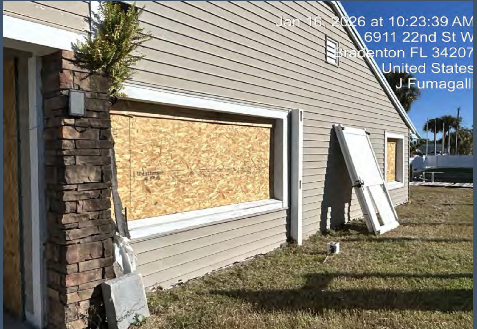
Boarded up windows on the side of the home.
