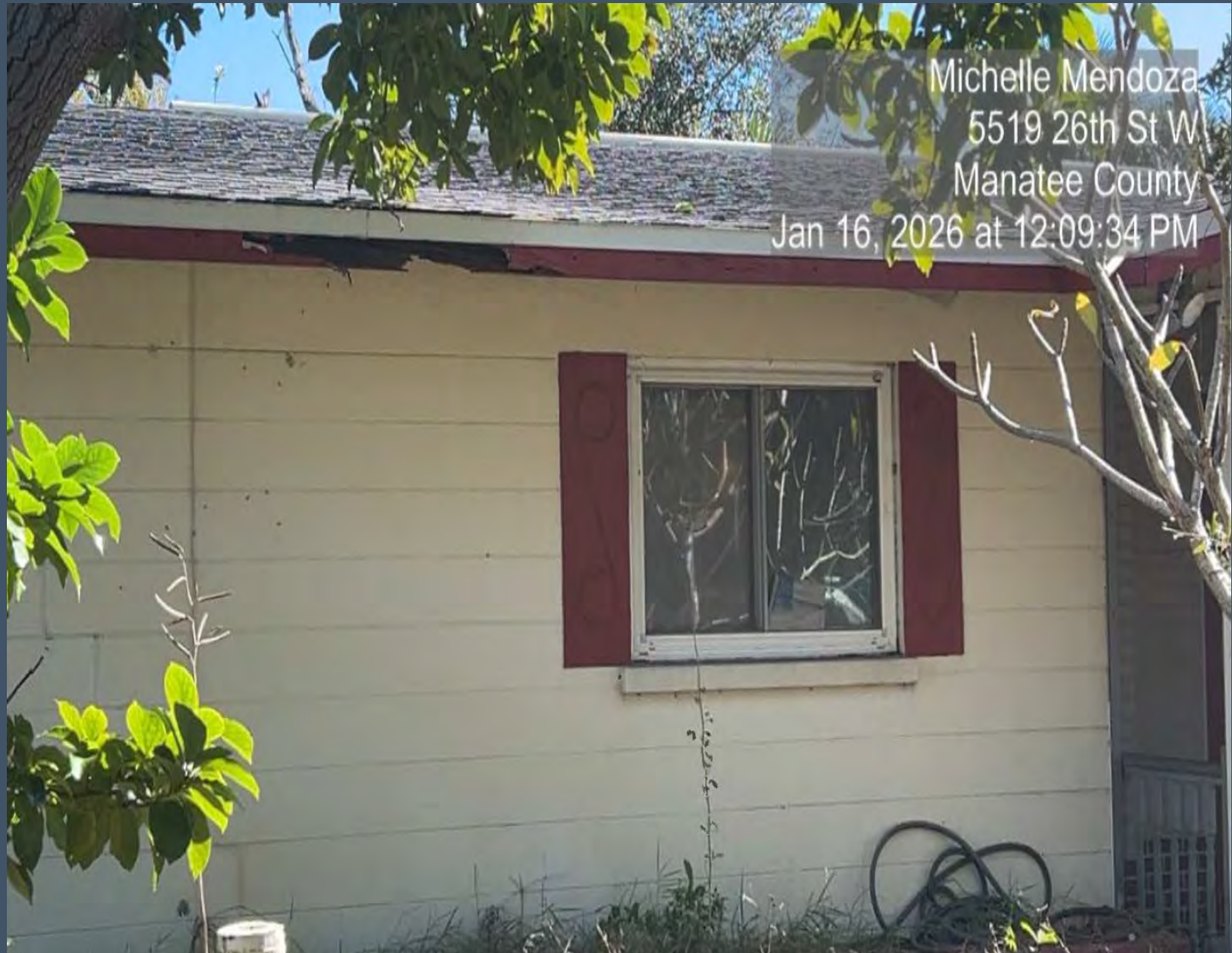
Photo of fascia still in disrepair.
