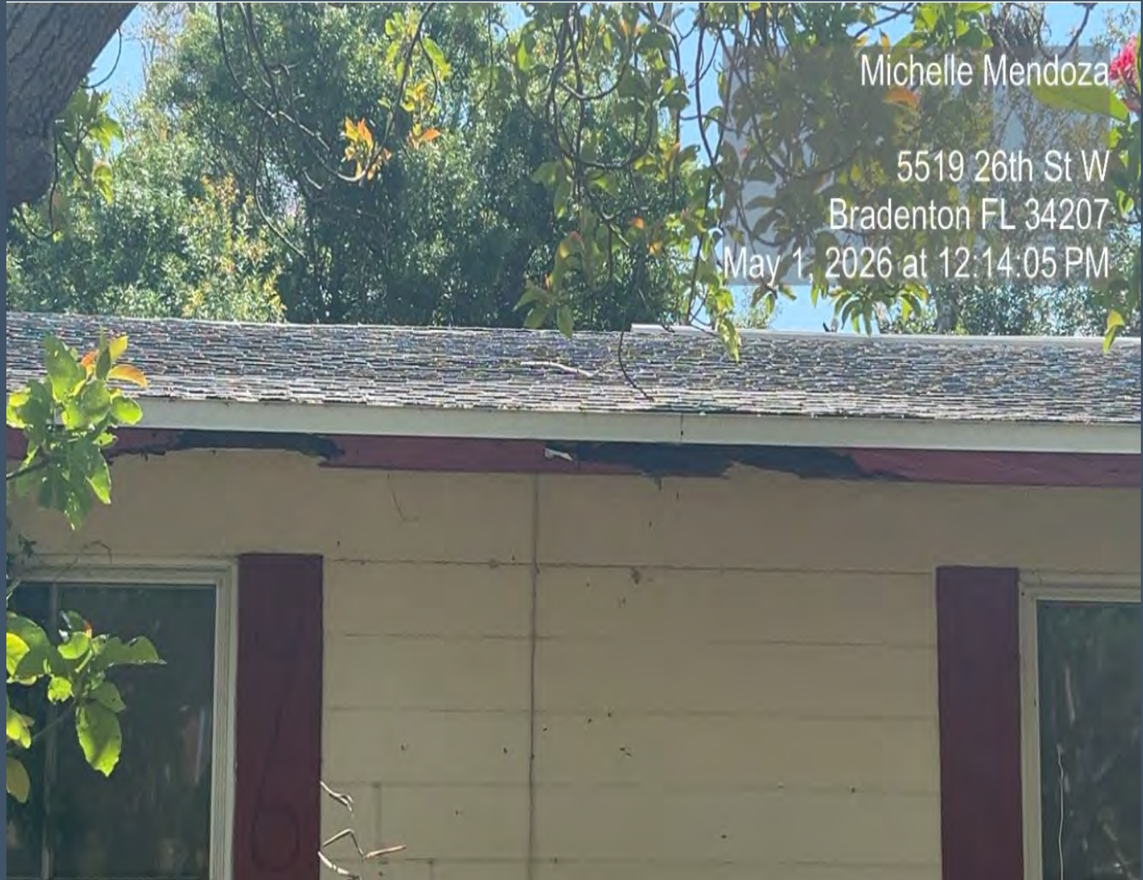
Photo of fascia still in disrepair.
