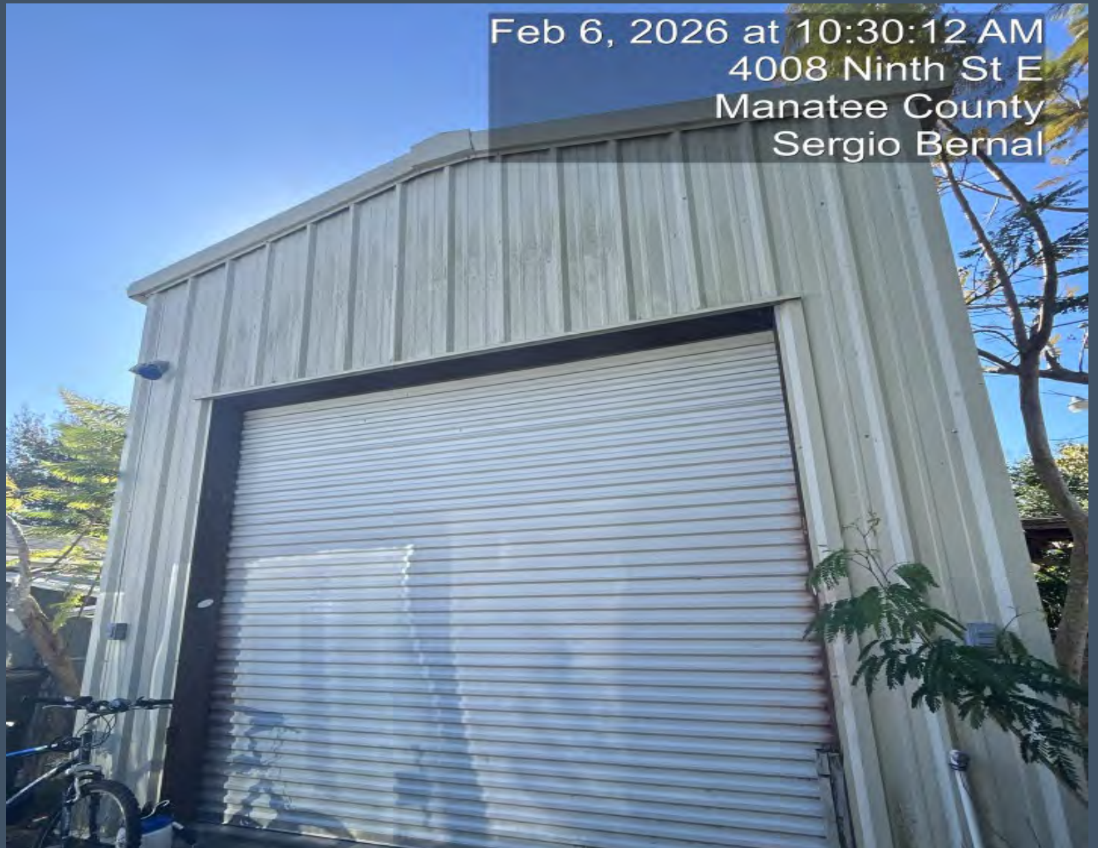
Photo of the unpermitted shed located in the rear of the property. (02-06-2026)
