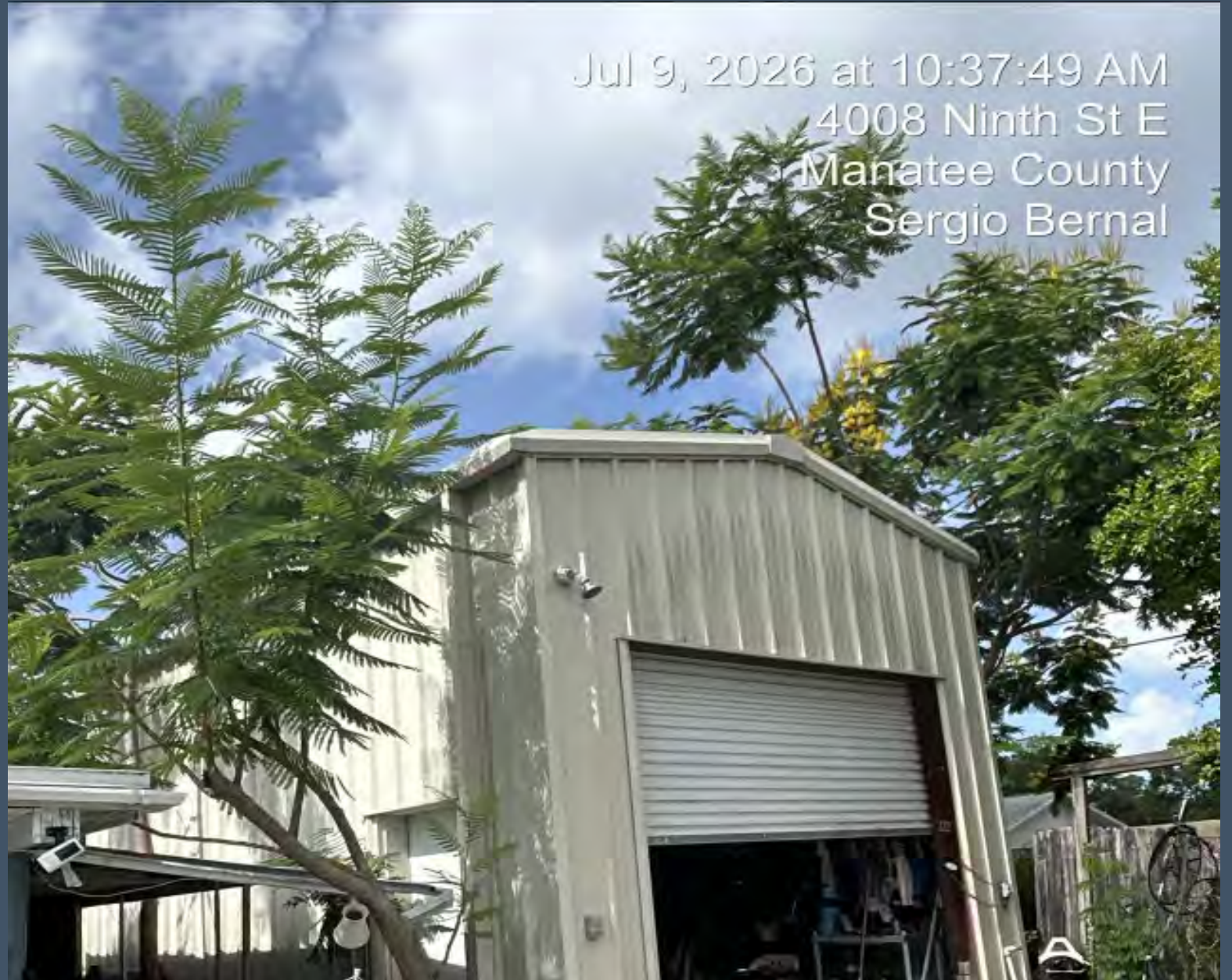
Photo of the unpermitted shed located in the rear of the property.(07-09-2026)
