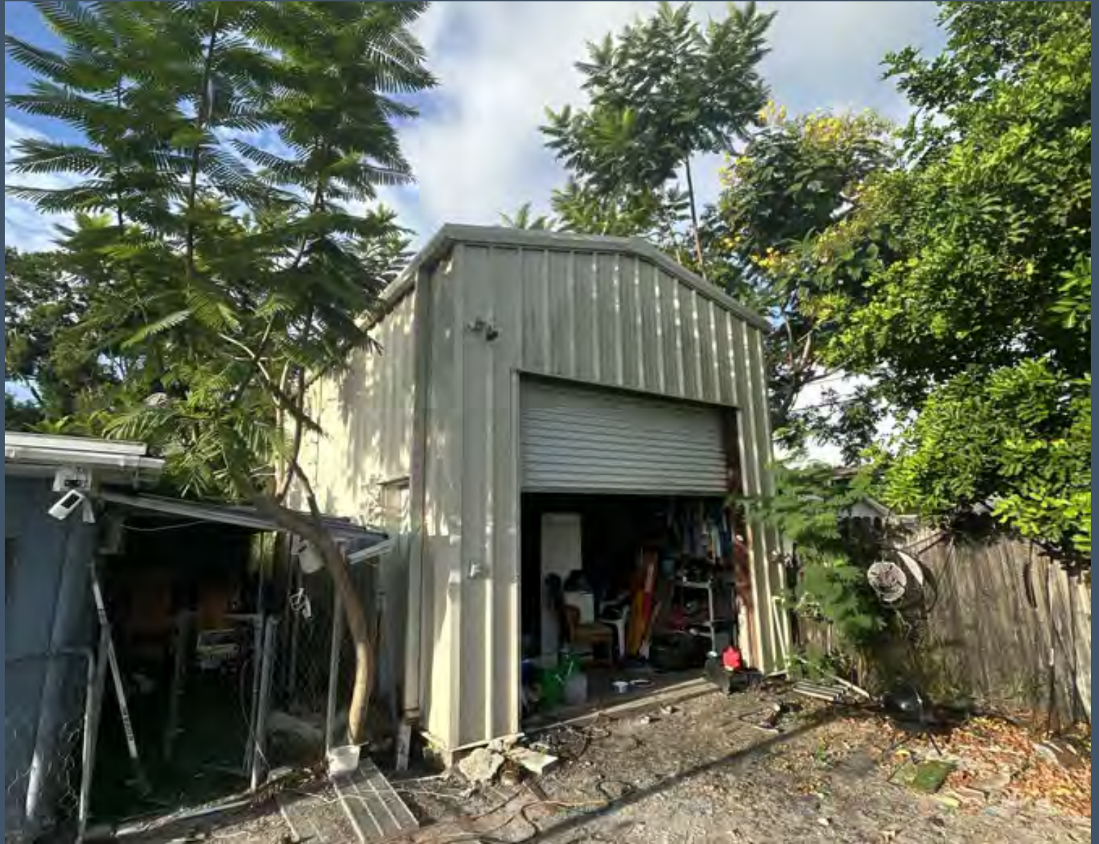
Photo of the unpermitted shed located in the rear of the property.(08-21-2026)
