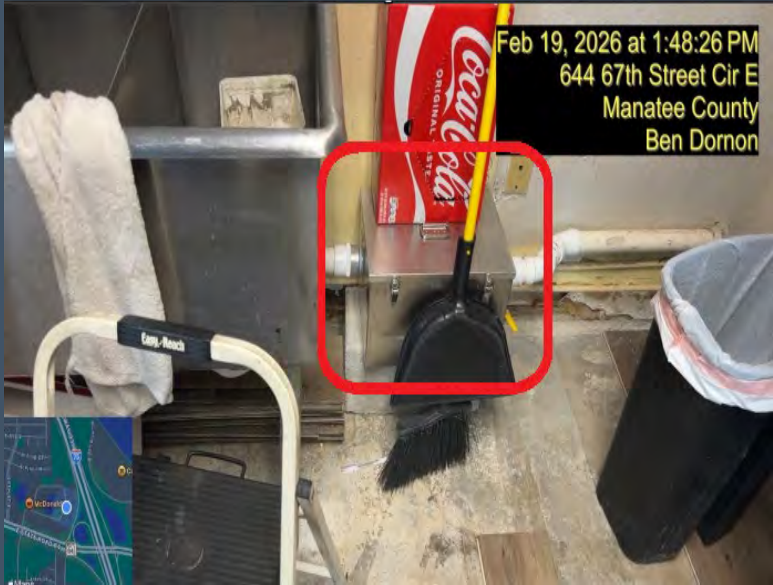
Unpermitted & unapproved grease trap
