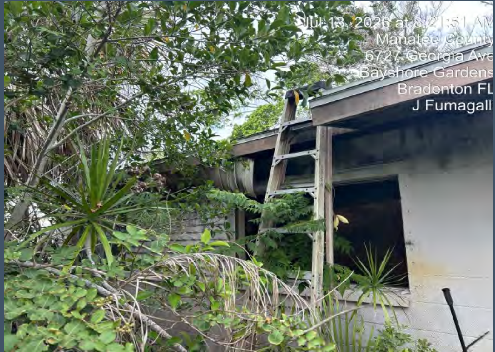
Photo depicts the roof in disrepair
