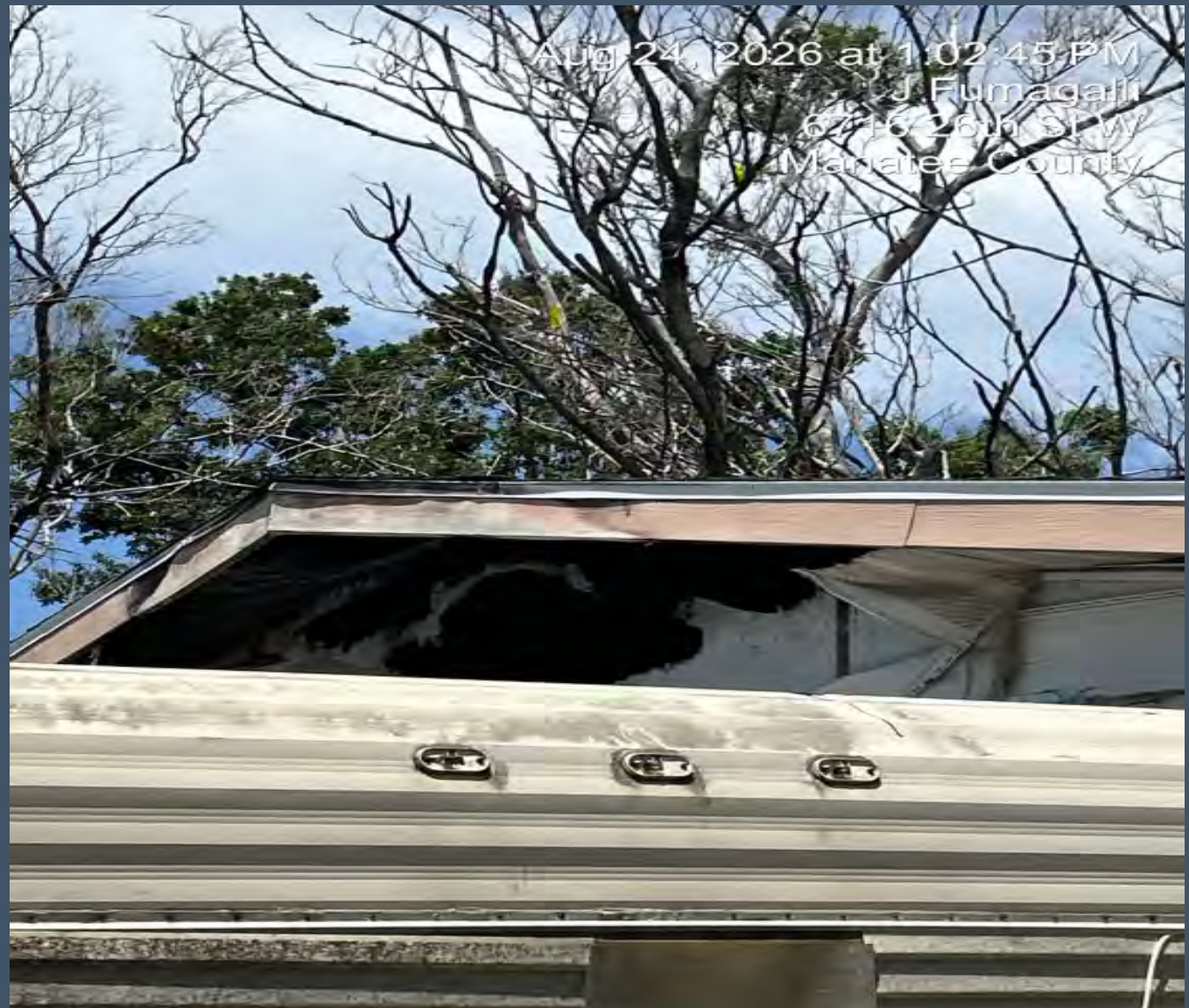
Photo depicts the roof in disrepair
