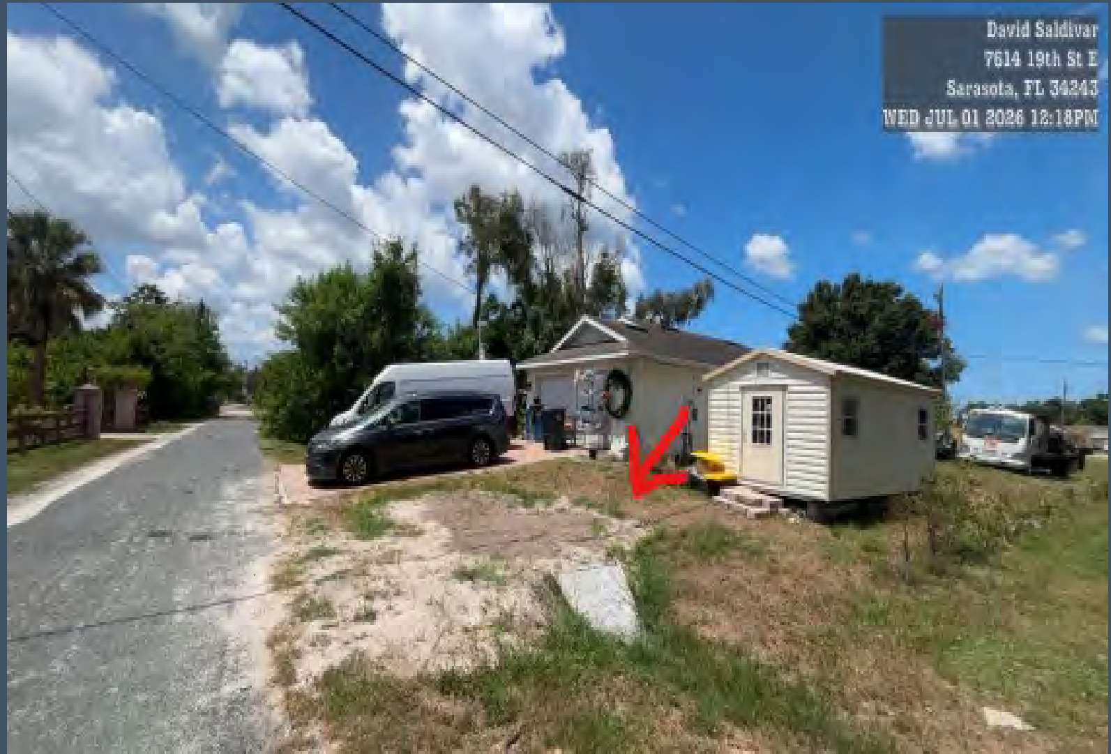
Picture depicts the culvert and dirt still in the ditch.
