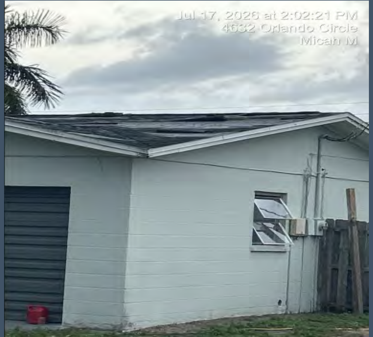
Missing roof tiles on July 17 th
