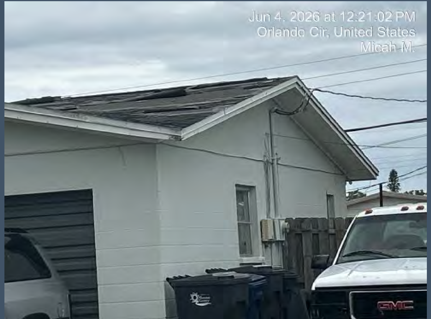
Closer view of missing roof tiles
