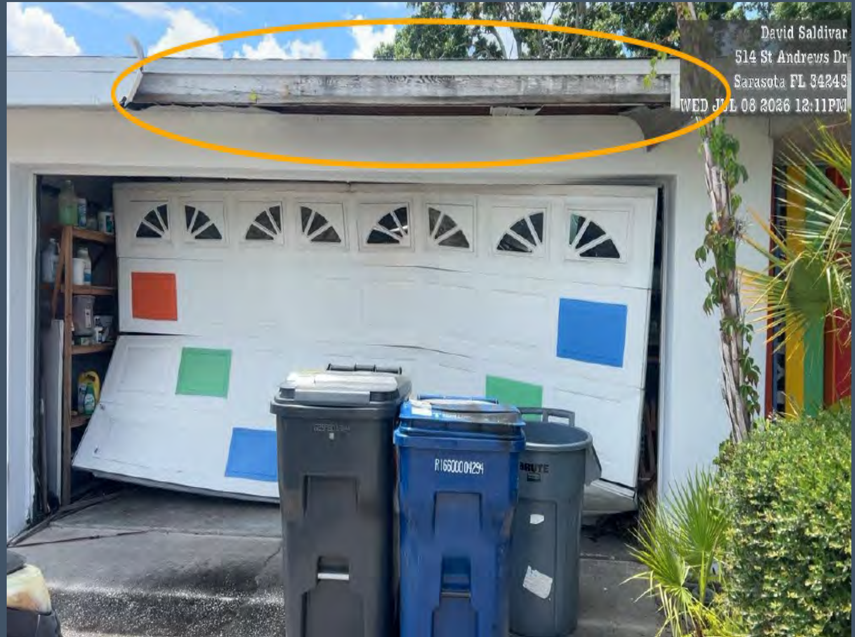
Picture is close up of damaged garage door and missing fascia and soffit.
