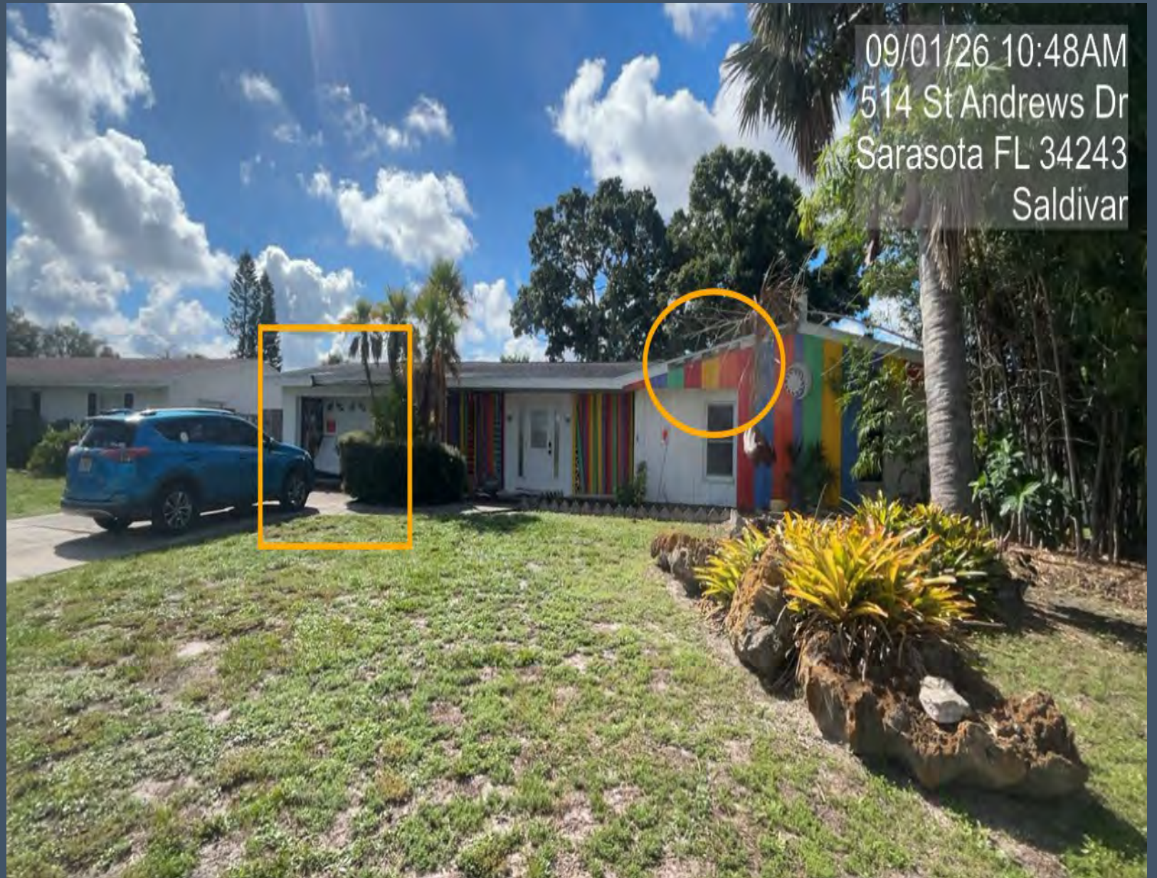
Picture depicting the front of the house showing the damaged garage door and missing soffit and fascia.
