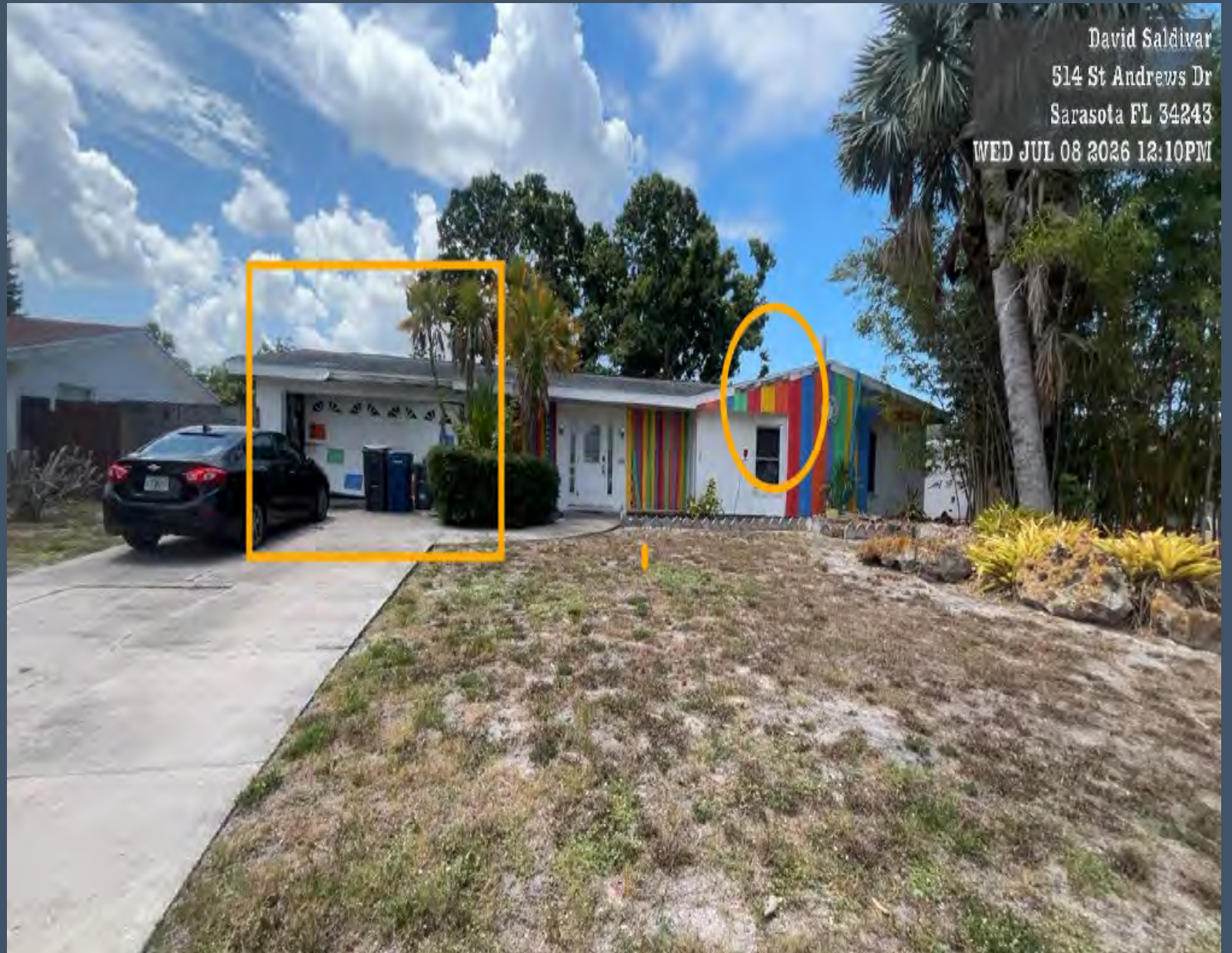
Picture of the front of the property depicting the damaged garaged door and missing fascia.
