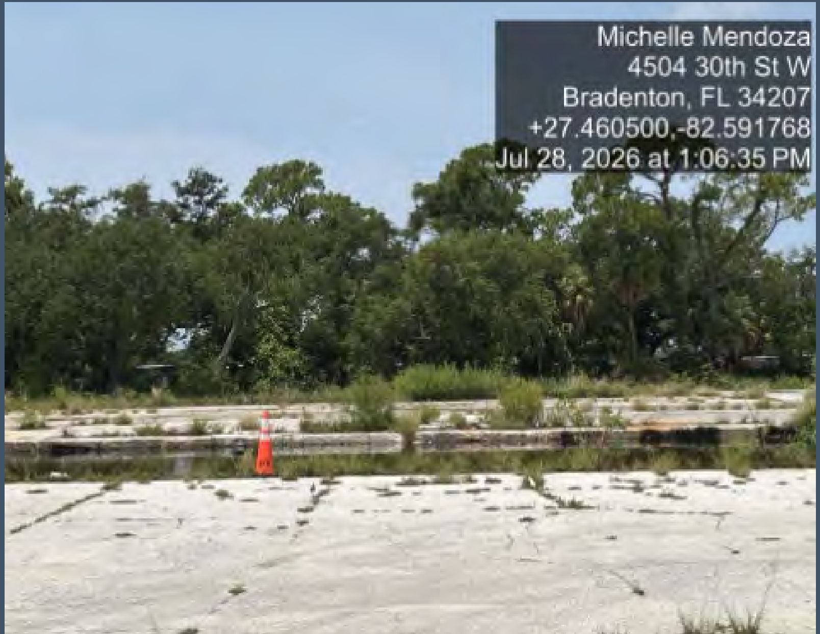
Photo of water in depressed loading dock.
