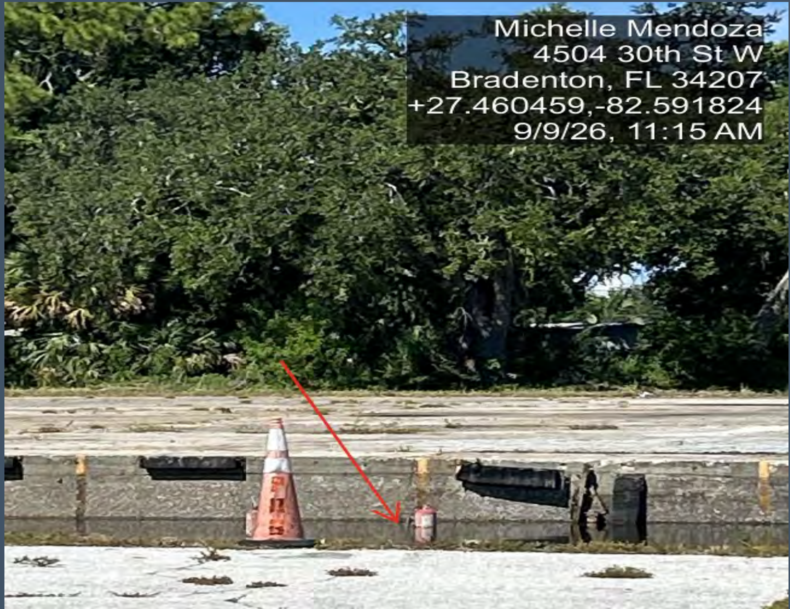
Photo of water still present in depressed loading dock at a different angle.
